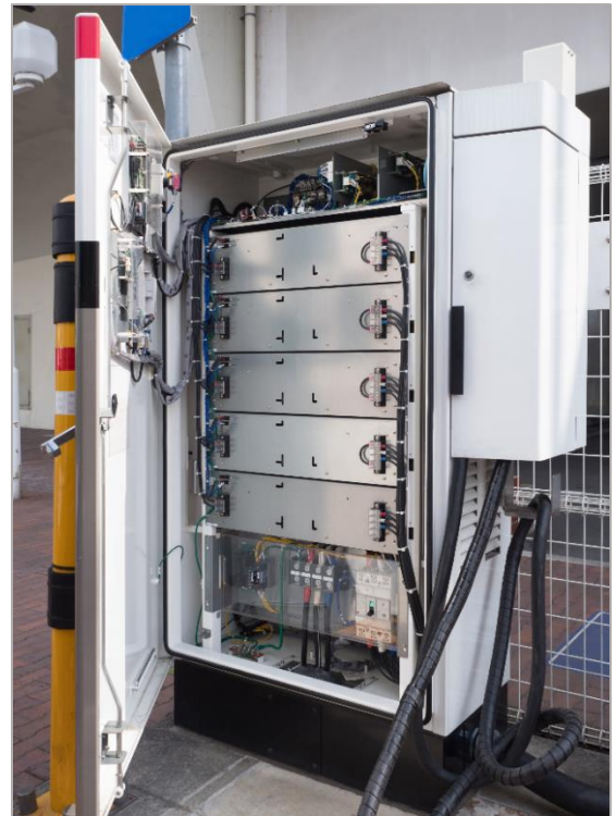
Cabinet for charging station
